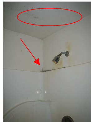
MBB shower, head leaks, moisture damage to wall
