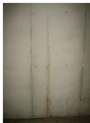
One of two cracks that should be repaired
