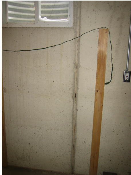
Crack north wall that should be repaired
