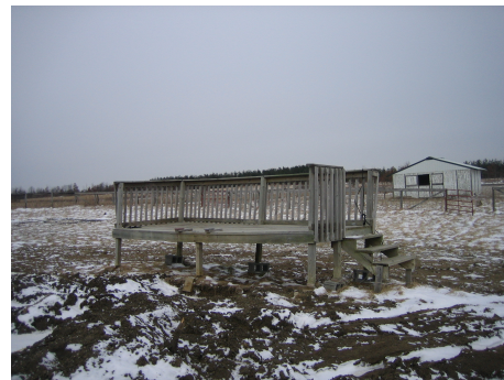
Recommend remove this deck
