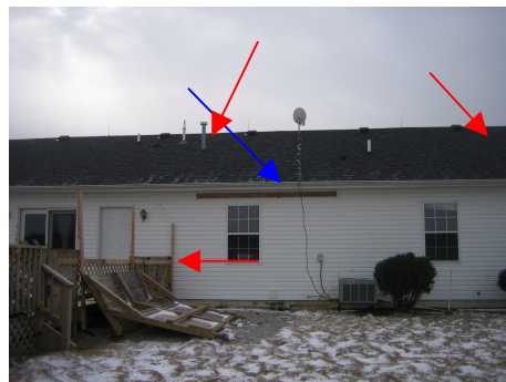
Repair siding, deck rail too low, spot repair roof, see next photo
