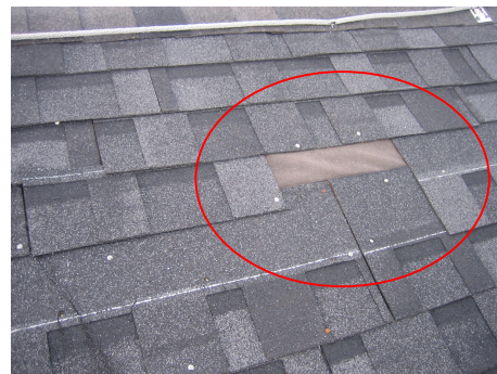
One of two repairs needed on roof
