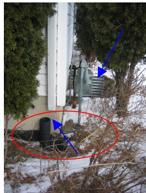
Fill in low spots, reconnect downspout, window well covers recommended
