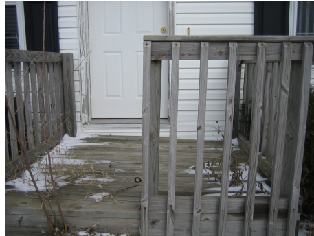
Front porch slopes, balusters loose recommend replace
