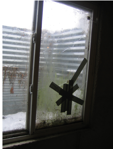
Broken window – basement east
