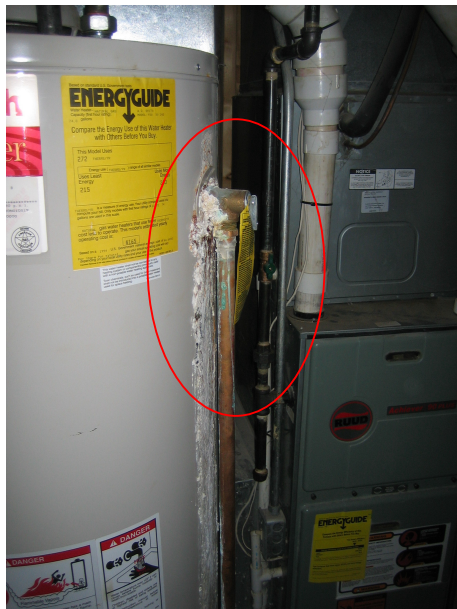
Water heater should be replaced
