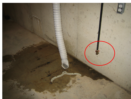
Result of water leak at sink in mud room Missing plug at gas line
